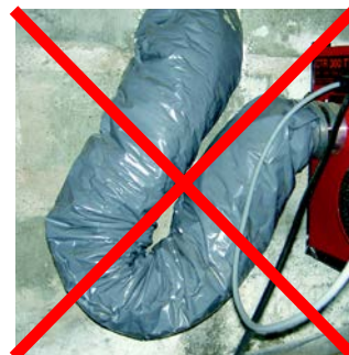
Feil montering, sterk bøy
